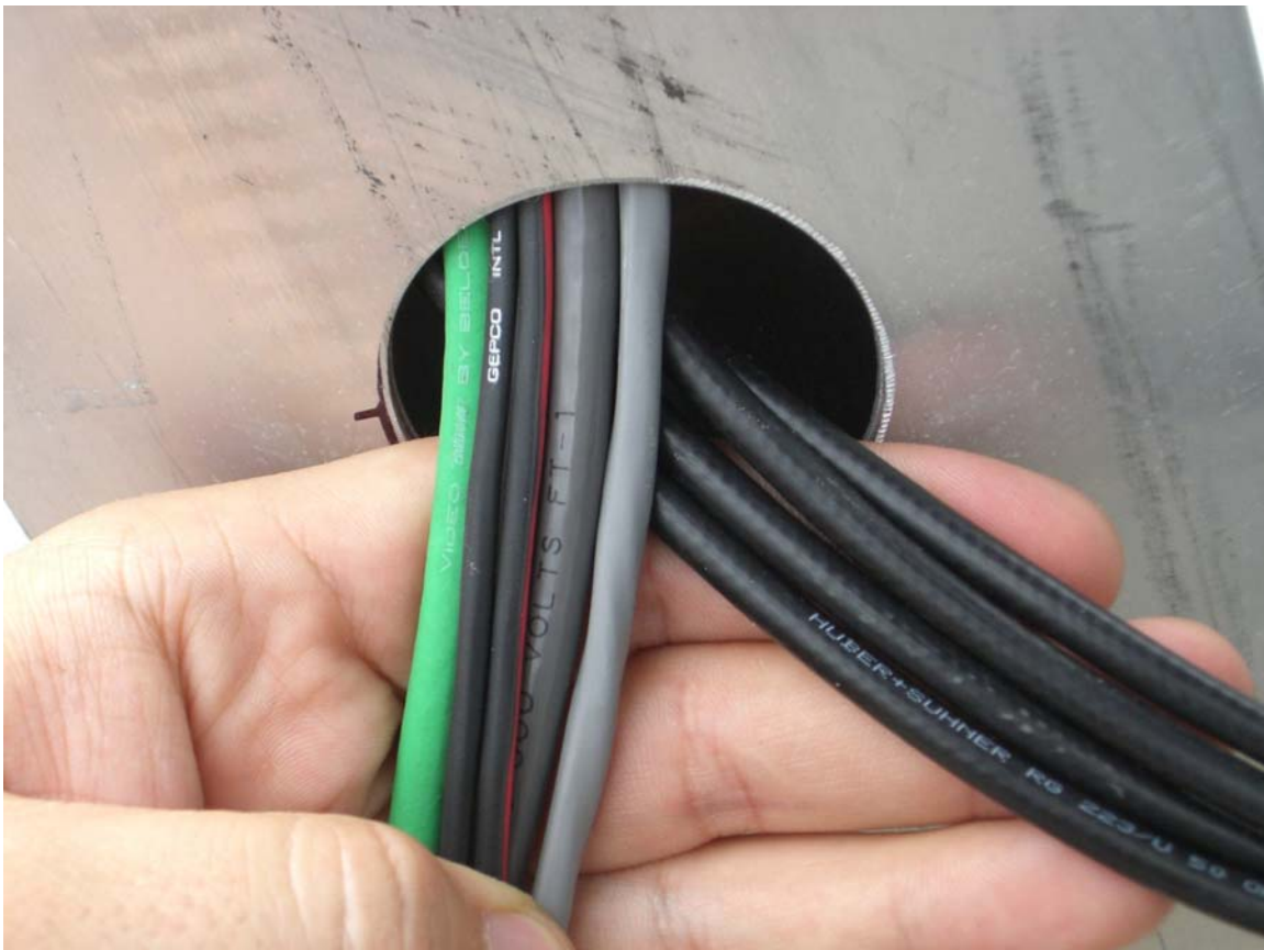
Figure 2: Cables required for TV and Telemetry
